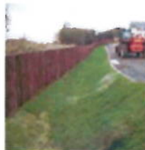
Grass Swale to attenuate & route surface flows
