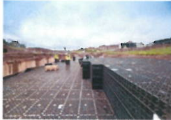
Modular Storm Tank (Carrowreagh, Dundonald, NI)
