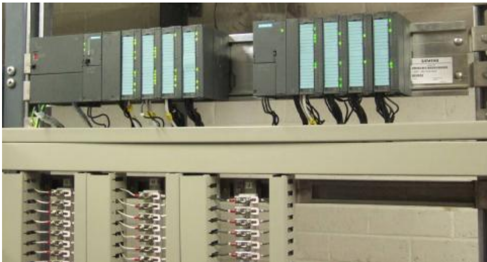
Figure 2.15 Siemens plc equipment at Londonderry Relay Room
