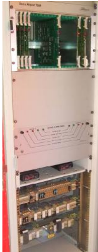
Figure 2.16 Westinghouse S2 TDM equipment at Londonderry Relay Room
