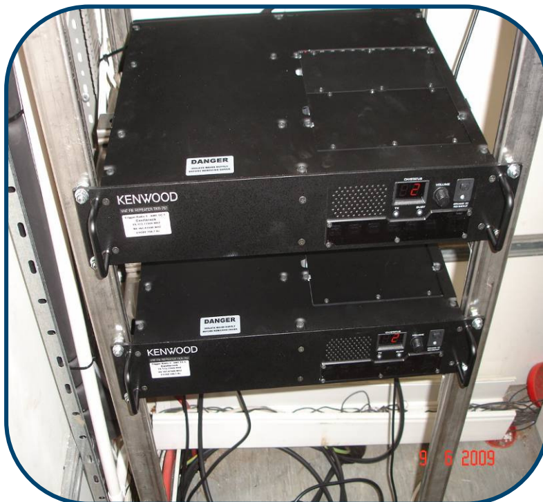
Figure 10: Kenwood VHF FM Repeater TKR-751 (Trigger Radio) - Castlerock
