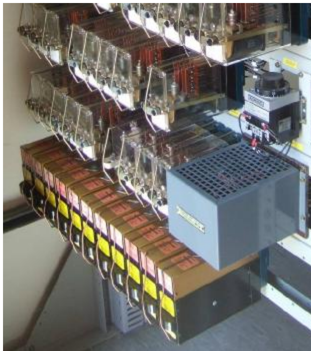
Figure 2.11 Redundant FDM equipment at Magilligan REB
