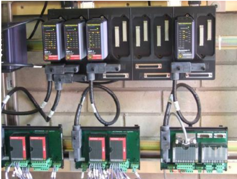
Figure 2.6 showing new Westinghouse S3 TDM mounted in Coleraine Relay Room
