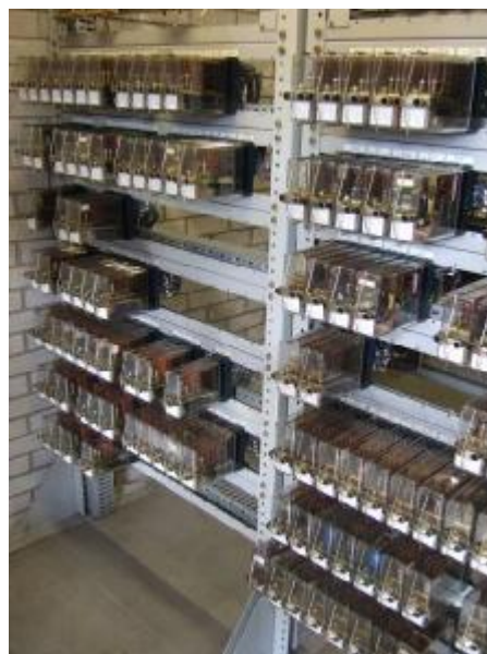
Figure 2.5 Available space within the racks in Coleraine Relay Room
