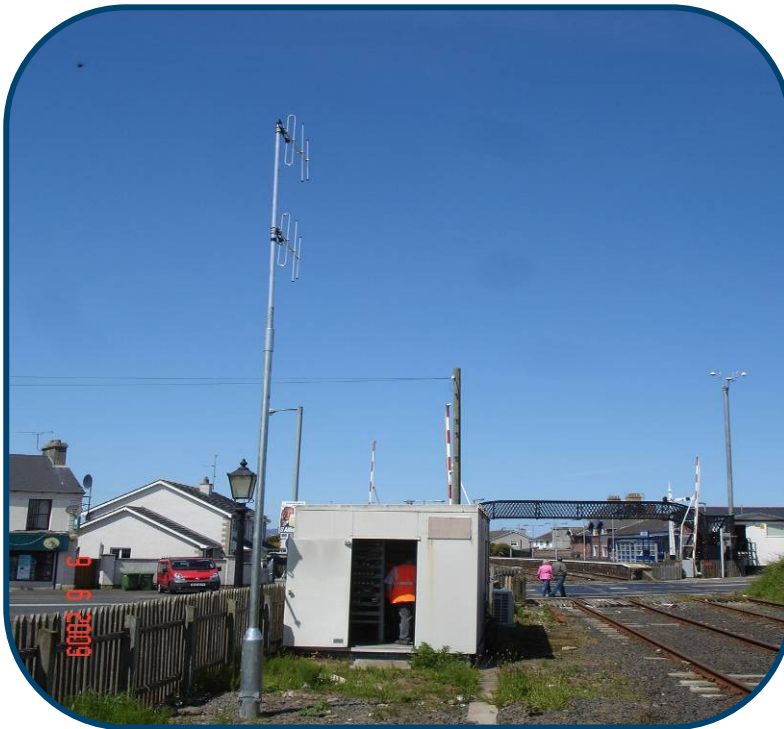
Figure 11: VHF Radio Antenna (Trigger Site) - Castlerock
