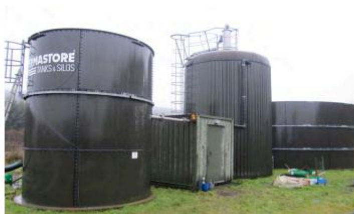
Installation showing input mixing tank on left, control kiosk, digester tank and post store
