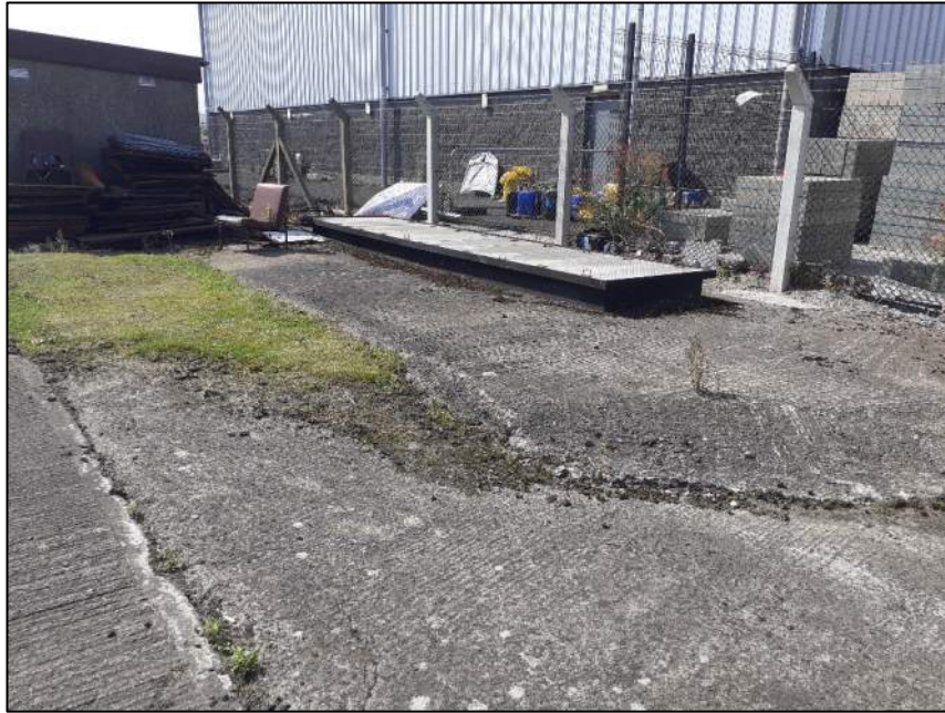
View of the cover over the Underground Storage Tanks (USTs) that capture the washings from the lairage.
