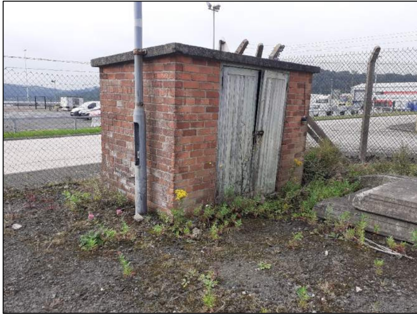
View of former electrical sub-station (ESS), now decommissioned, at the southern boundary, adjacent to the DAERA site boundary.
