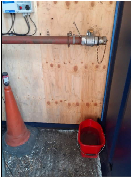
View of diesel tank fill point pipe and spill bucket below.
