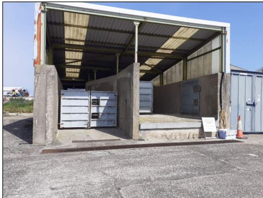
Entrance to the lairage with grating to capture run-off along the front.
