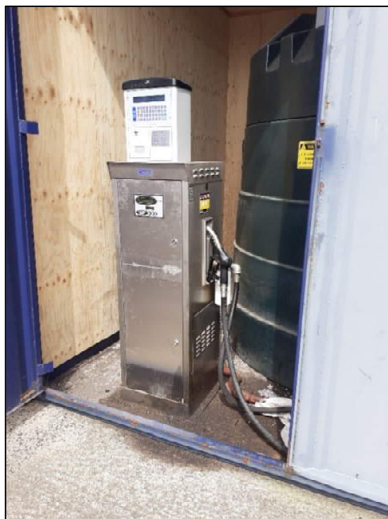
View of diesel tank and pump inside container with staining on ground.
