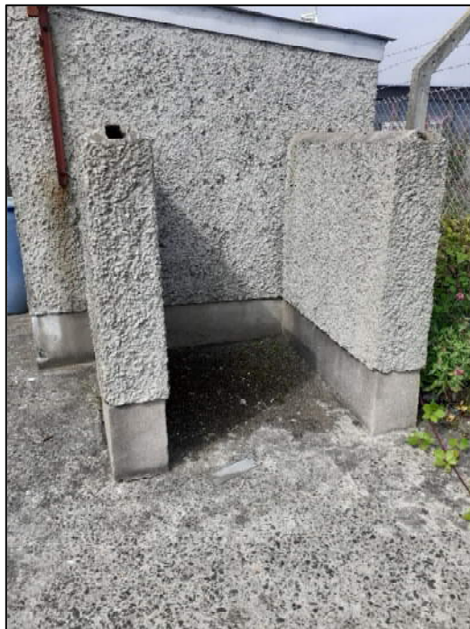
External possible tank location adjoining the pump house to the east of the former garage, with the vehicle inspection ramp to the south.
