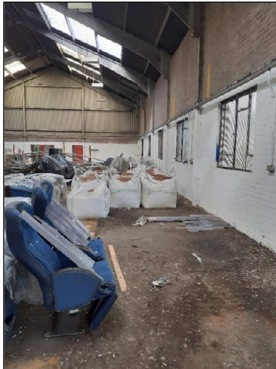
View inside the former garage, now used for storage with oil staining remaining on the concrete floor.
