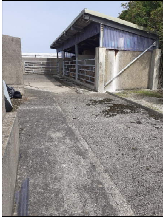
View of straw storage area to east of the lairage with drainage gully's and grates.
