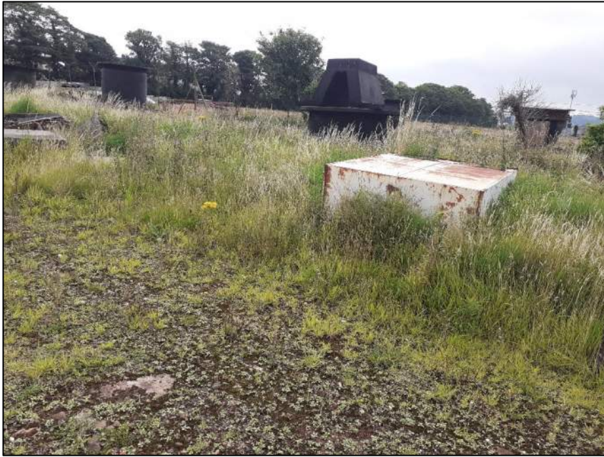
View of old empty rusted metal oil tank with fenders to the rear in the northern area of the site.
