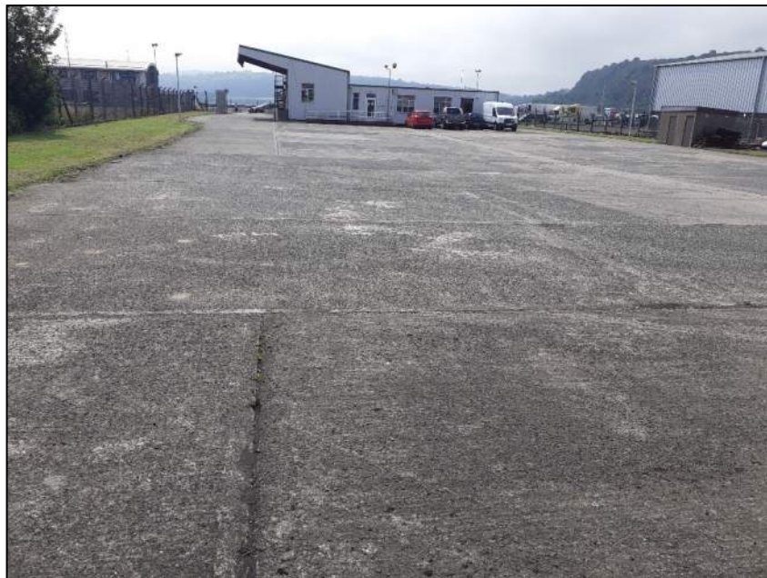
View from northern end of the DAERA site outside lairage, looking south towards the inspection office and gantry.
