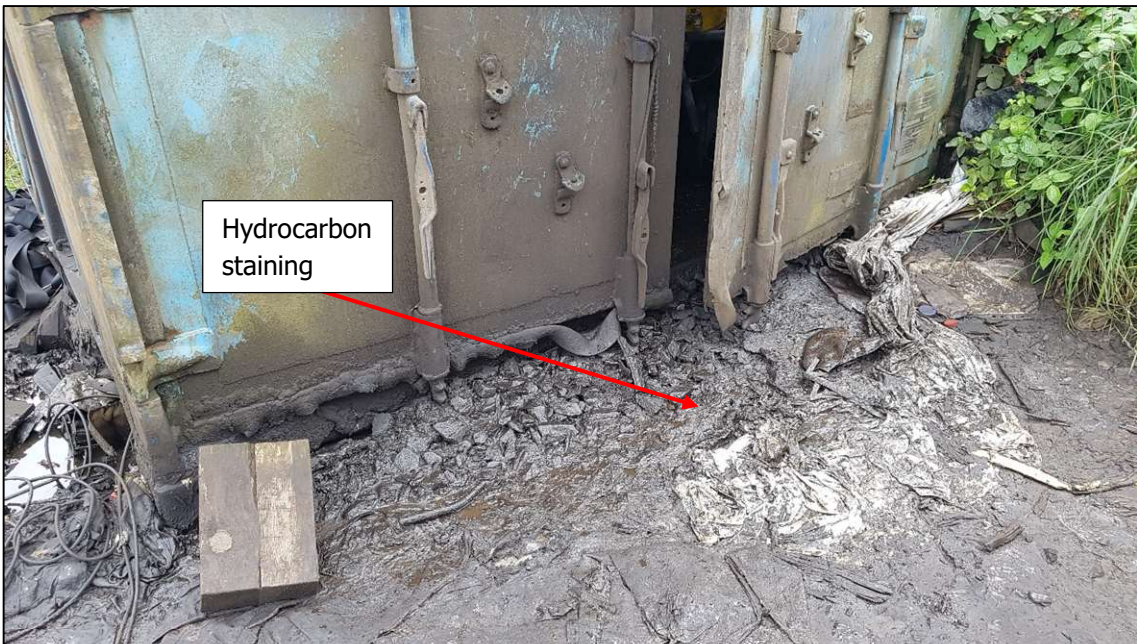
View of the electric substation located in the northern eastern corner of the site, adjacent to the northern boundary.
