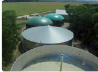
The 30 day fermentation process taking place with in these tanks delivers methane to the gas engine
