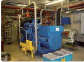
1600 KW biogas CHP plant room
