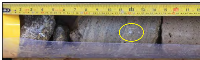
Fig.18 Steel bar ( circled ) embedded in gunite in core 4.
